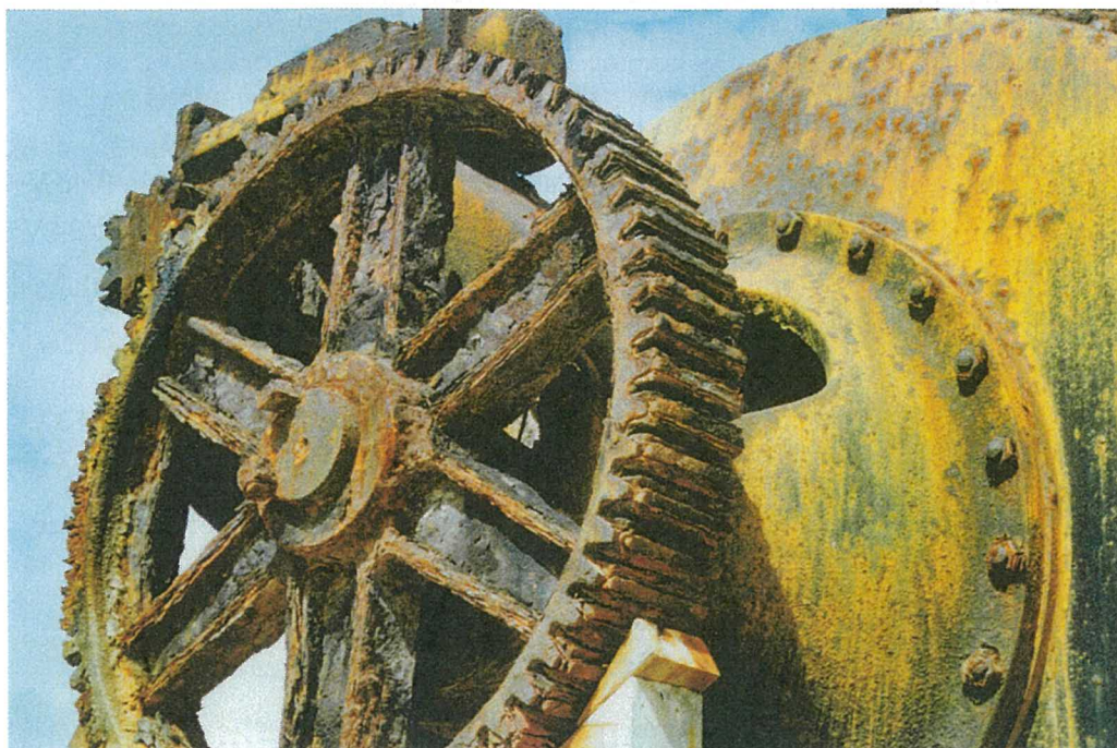
Rust is slowly destroying this abandoned whale blubber boiler on Norfolk Island
